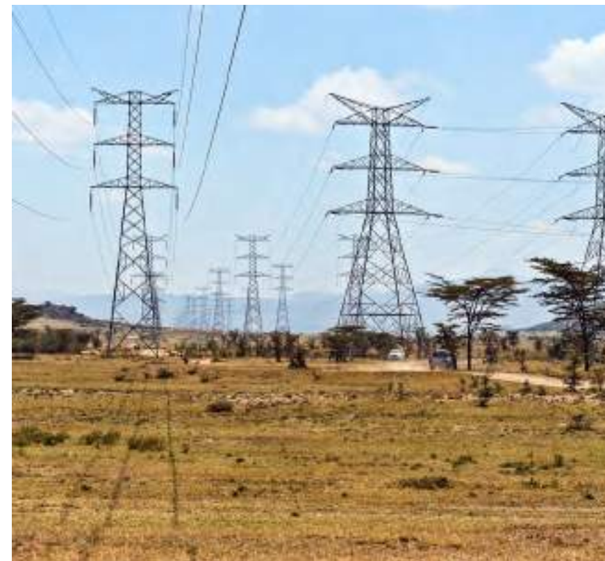
Strengthening and modernizing Africa's electricity grid is a key enabler of a just transition and should be a major policy focus.
