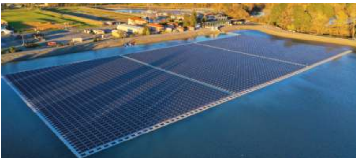
Floating PV site in Windsor.
