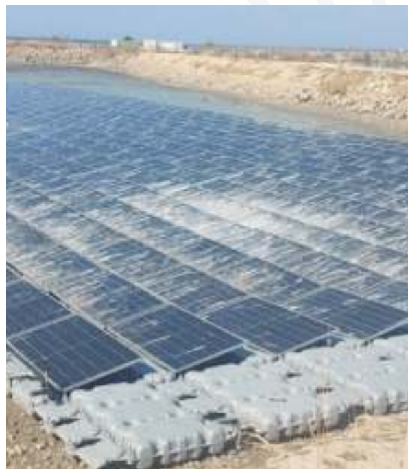
Bird soiling - in white - can be seen on the PV panels.
