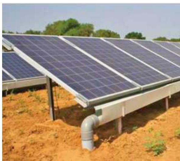
Central Arid-Zone Research Institute (CAZRI) Agrivoltaics plant, Jodhpur, Rajasthan. © CAZRI.
