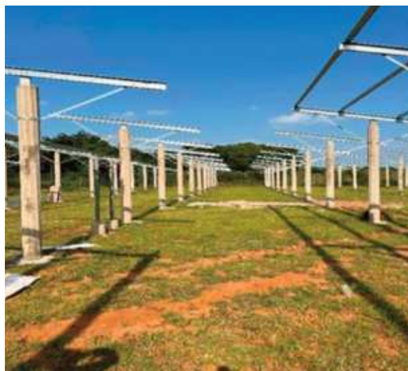
Phase 2, Indra Solar Farm, Agrivoltaics plant, Tikamgarh, Madhya Pradesh. © Khare Energy Private
