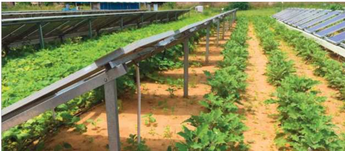
Central Arid-Zone Research Institute (CAZRI) Agrivoltaics plant, Jodhpur, Rajasthan. © CAZRI.
